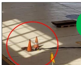
Ground Power Port with safety cone
