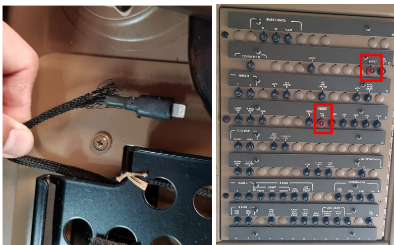
Gambar.(a) Electrical outlet P-EFB fraying; (b) Maintenance Overhead Panel P11
